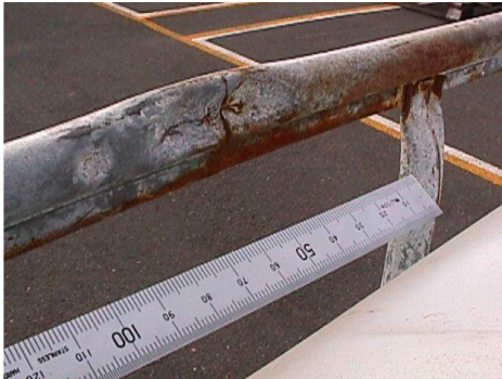
Pic 5: Rust is longer than 25mm (1 inch) - Not acceptable
